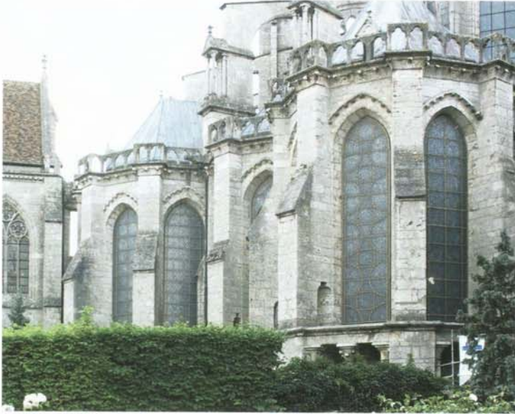
Fig. 7. Exterior view of choir chapel windows with thermoformed protective glazing, installed 2008, Chartres Cathedral (photo: author)
